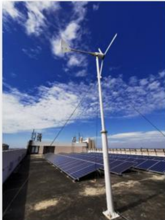
Wind turbine generator
